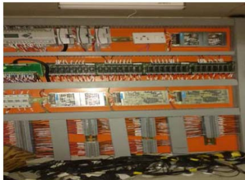
Figure 9: Control Panel Wiring
