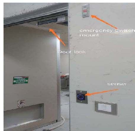
Figure 12 : Actual System Installation
